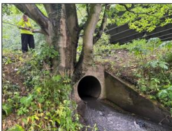
This is the outfall from the M6 motorway in Lancashire discharging into the River Darwen. It discharges every time it rains, causing river pollution.
