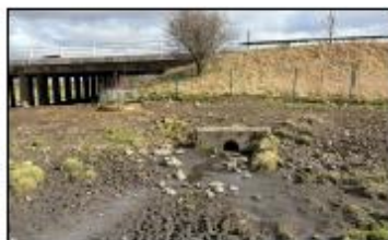
This outfall off the M6 discharges into the River Lune at Tebay which is a salmon fishery.
